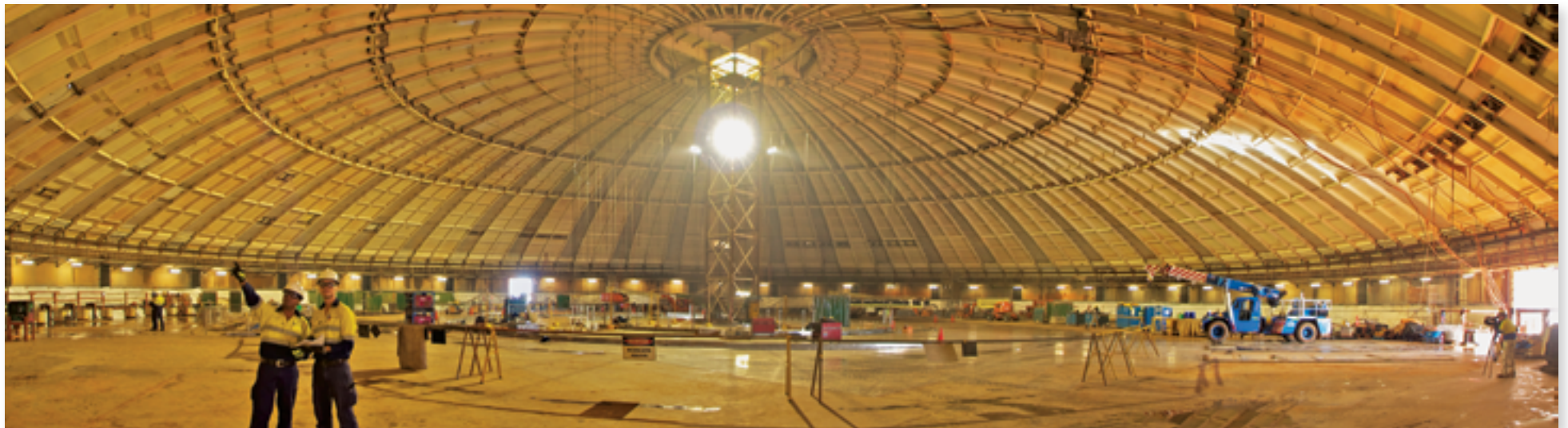
Inside one of the LNG storage tanks which will hold 180,000 cubic metres of LNG (photo courtesy Chevron Australia)
