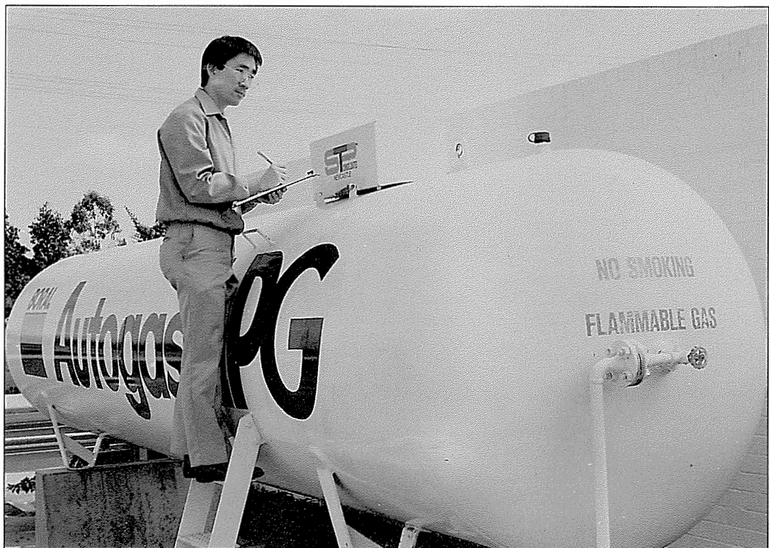
Inspector Lawry Lim conducts an inspection of an autogas LPG installation at a metropolitan service station.
