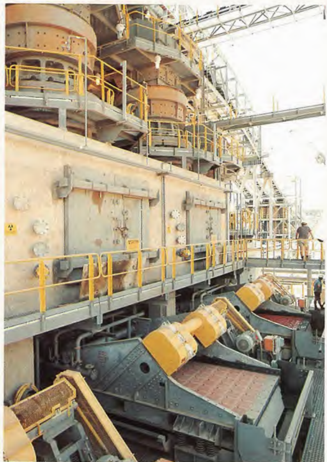
Tertiary cone crushers and screens at the Argyle Mine treatment plant (November 1985 photo, reproduced with permission of Argyle Diamond Mines Pty Ltd).
