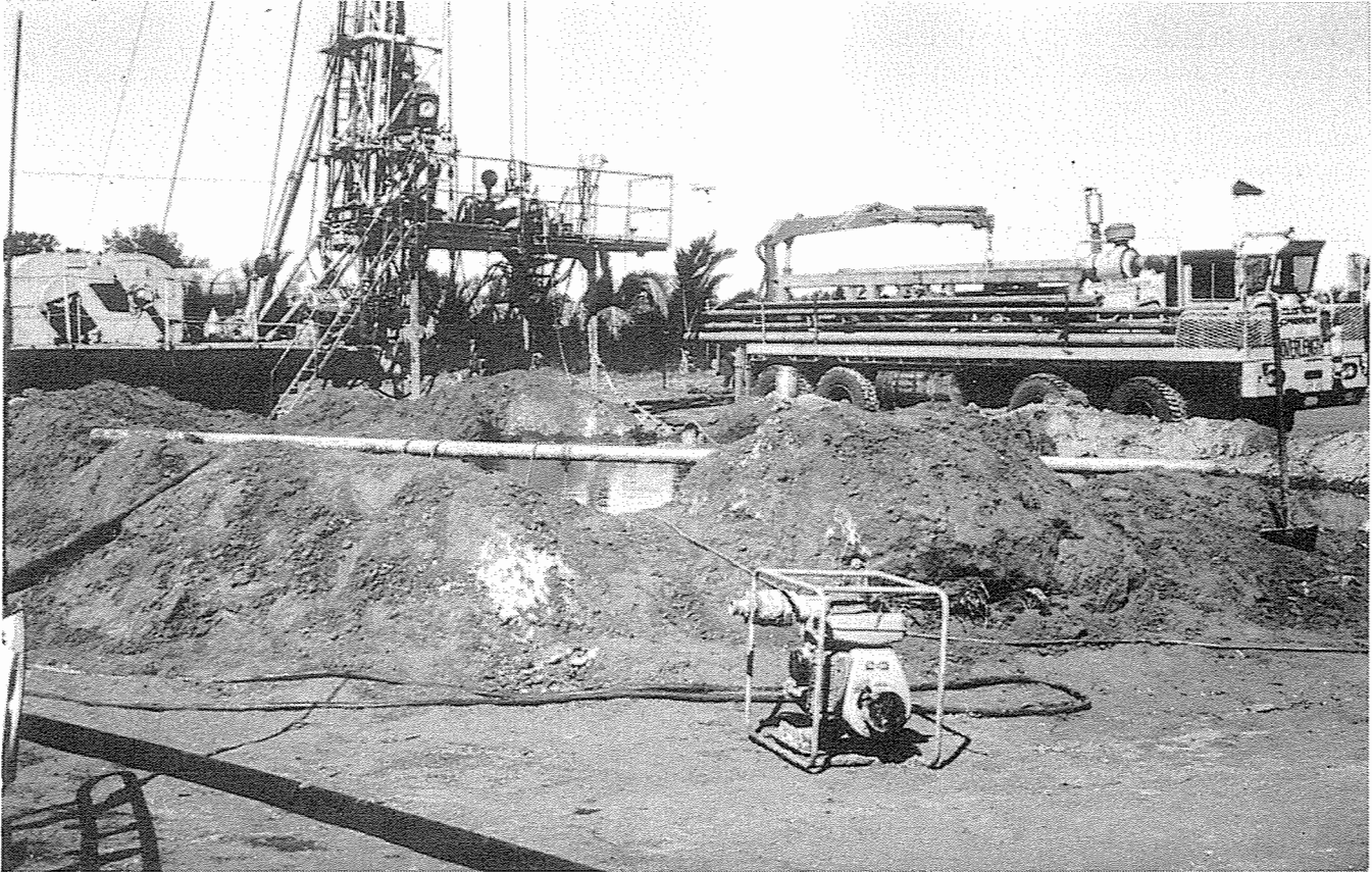
Drilling the 500m-deep privately-funded artesian bore which produce a flow of 500m 3 per day of slightly brackish water which will be desalinated for irrigation of horticultural land.
