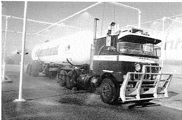
Water fire protection at the tanker loading facility at Kleenheat's Kwinana LP gas installation. This protection meets the requirement of Australian Standard 1596.
