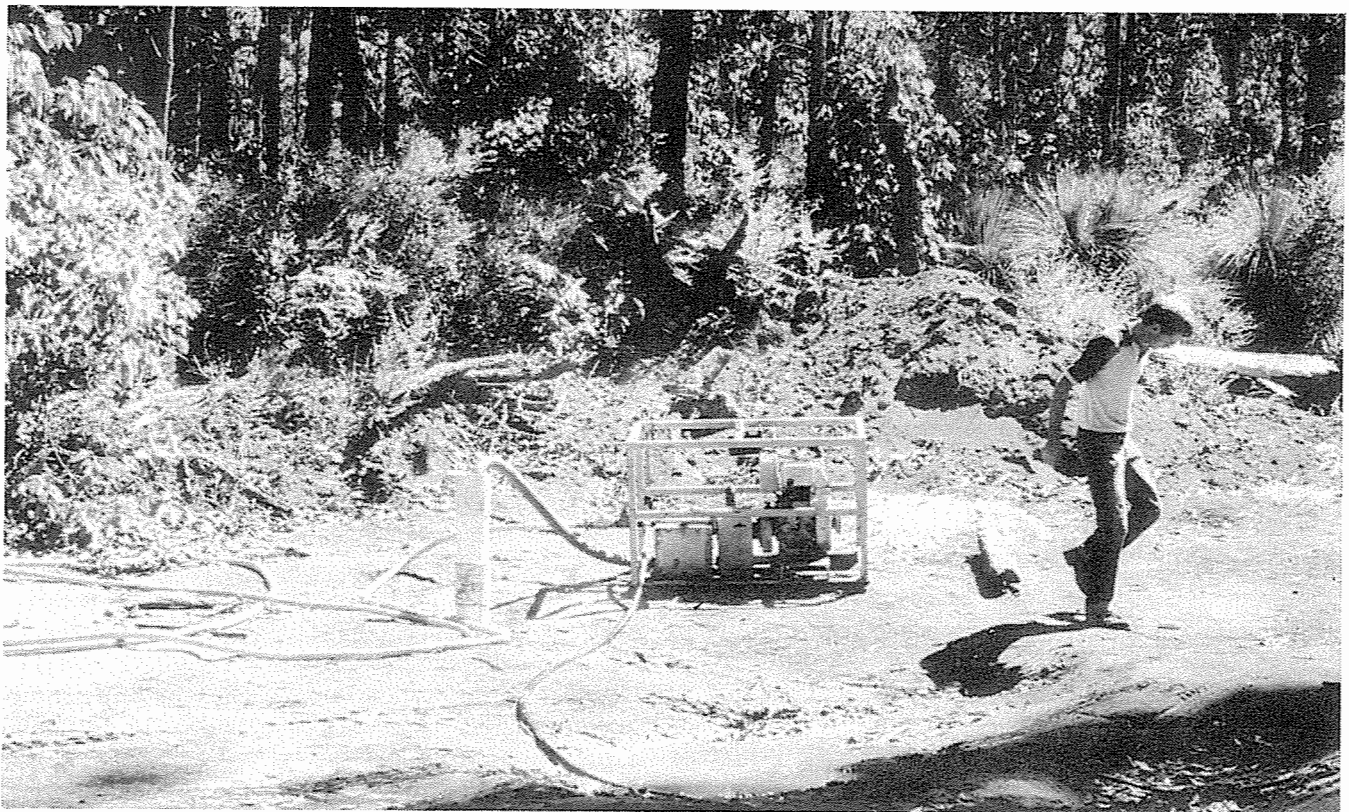
Pump-testing groundwater at the Harris River damsite to determine permeability of foundation rocks.
