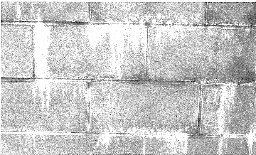
Efflorescence on concrete masonry caused by the movement of lime from the mortar joining blocks
