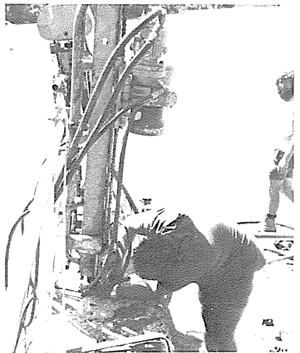
Core drilling to test ongoing stability of the Bickley reservoir concrete gravity dam
