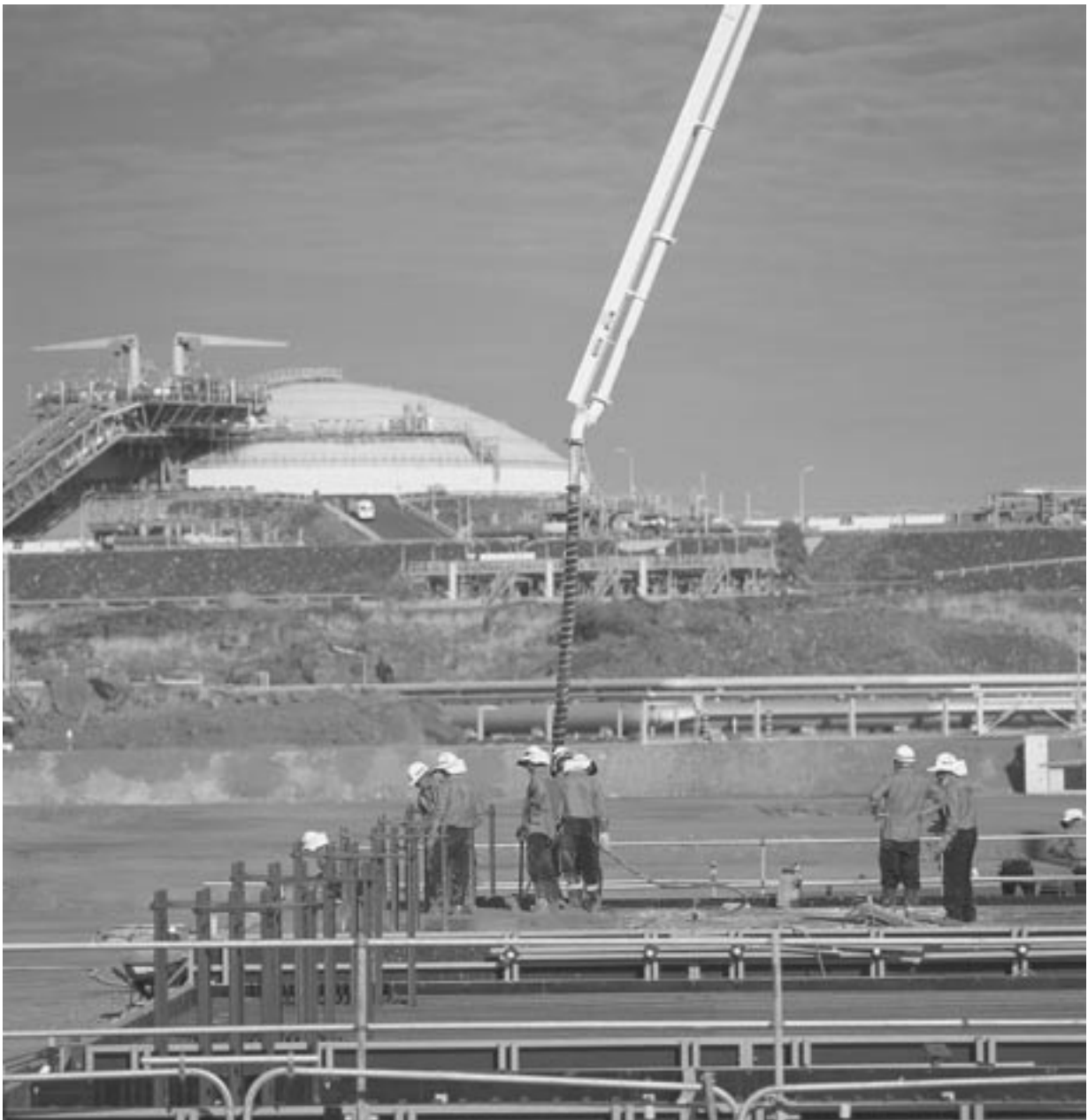
Construction of the fourth LNG train as part of the North West Shelf LNG project is a significant investment currently taking place in the Western Australian resource sector.
